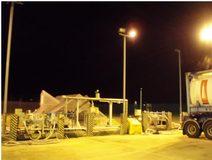
High pressure Sodium lamps in floodlights providing both operational as well as security lighting.
