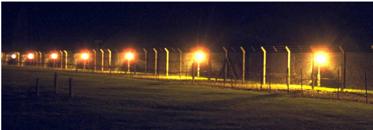
Glare Lighting installed to cover a section of a perimeter
